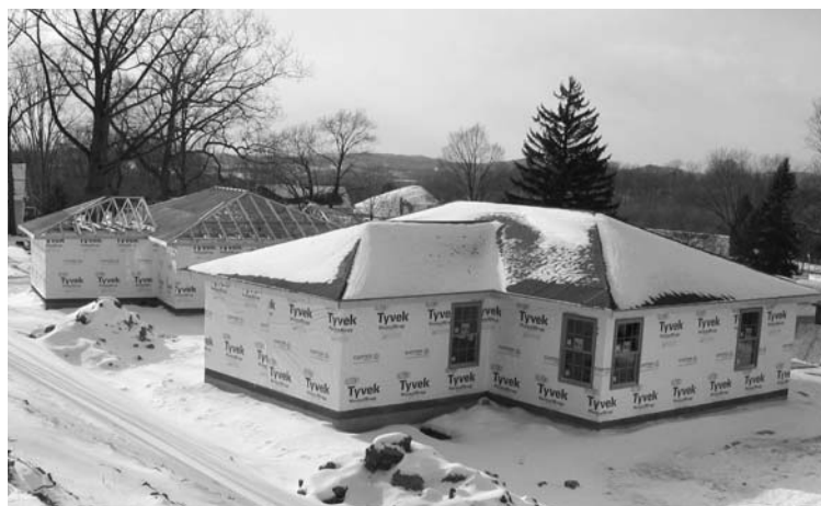
Construction of the all-season cabins progresses during the winter. Each cabin can accommodate up to 20 people.
